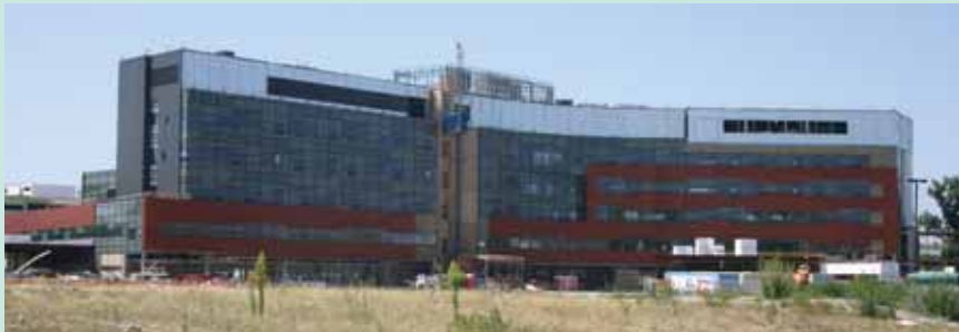
Construction progress on the new hospital continues. The main entry canopy is to the right, and the Emergency entry canopy is to the left.
