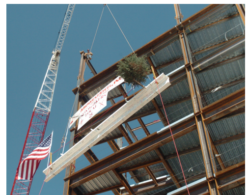
The final steel beam is lifted into place. “Topping off” dates back to 700 A.D., when Scandinavians topped off construction of new halls with grain. Over the years, grain was replaced with evergreen trees and, in America, the addition of a U.S. flag. The tree symbolizes new life and growth, a job well done and a new beginning.
