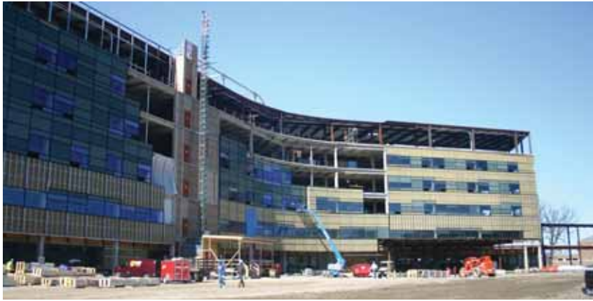
Construction on the east side of the new hospital building; on the far right is the structural frame of the two-story connector to the present medical center building.
