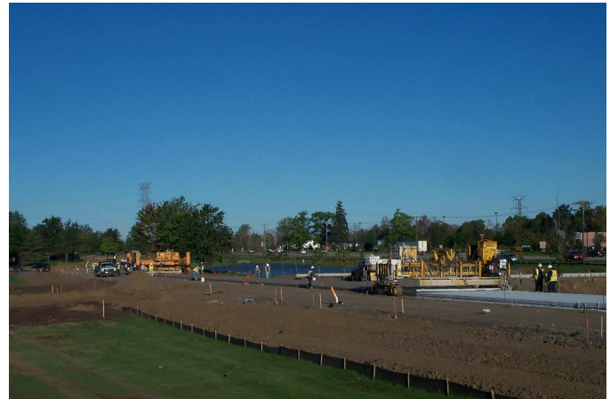
Concrete paving in progress along the north section of the Ring Road.
