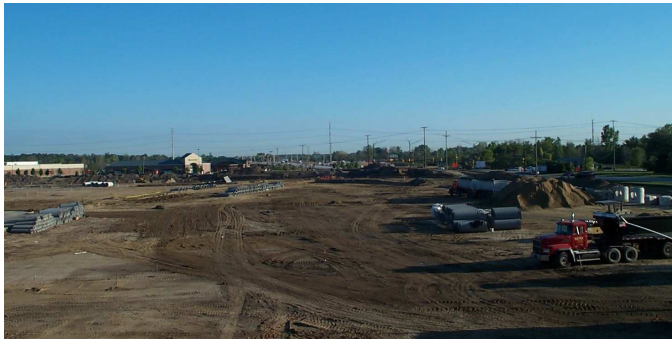
Rough grading and underground utilities in progress at the East Parking Lot.
