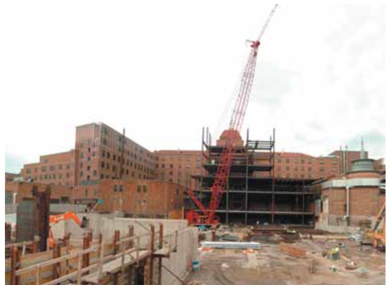
The structural steel skeleton of the six-story North Pavilion is scheduled to be completed by the end of Fall 2006.
